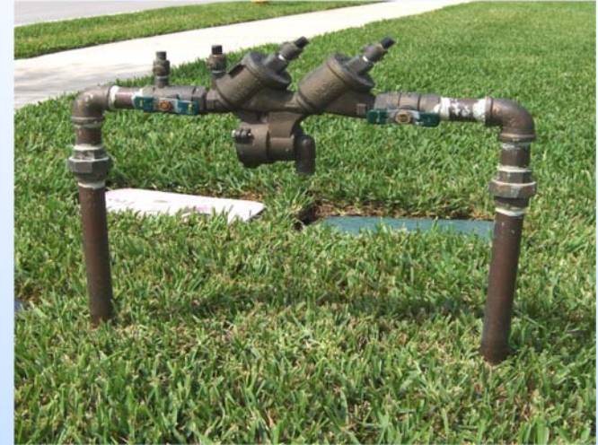
A typical residential backflow preventer.
