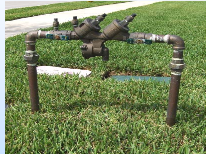
A typical residential backflow preventer.
